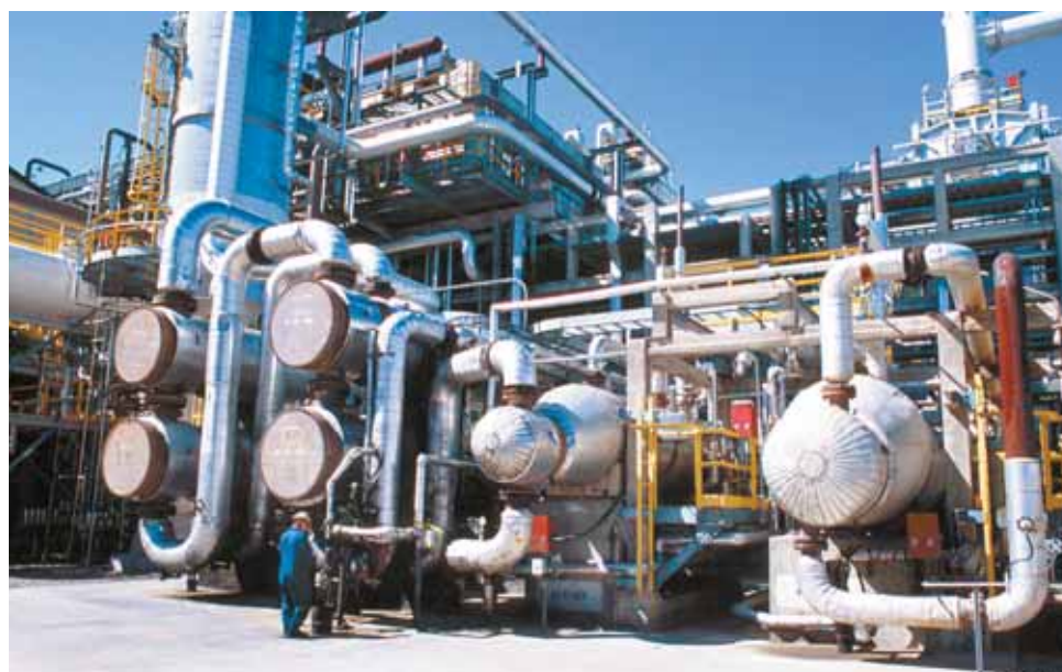
Husky's Lloydminster Upgrader draws heavy oil feedstock from the Lloydminster and Cold Lake areas and processes it into high-quality, low-sulphur synthetic crude oil feedstock for refining into premium transportation fuels used in Canada and the United States. Photo provided by Husky Energy Inc.
